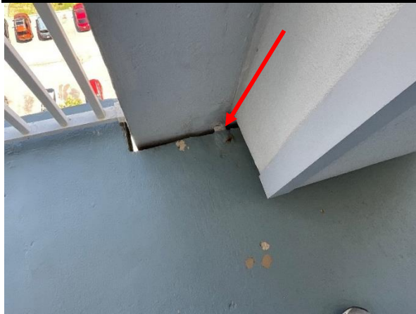
Photo 13 East Elevation – Common Walkways – Floor 11 – View of corroded knee wall tab – Typical.
