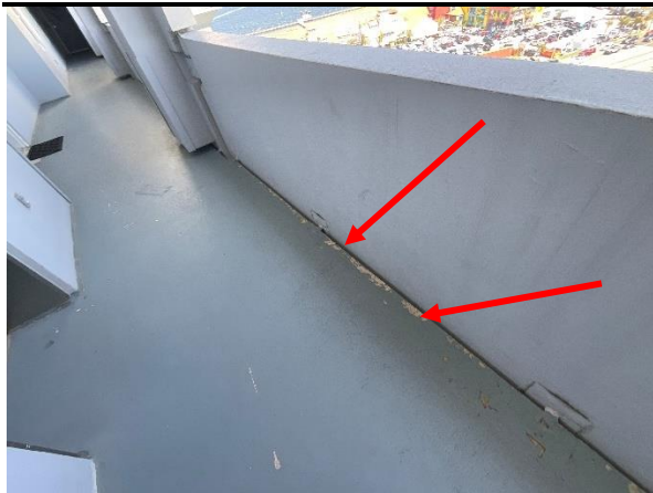
Photo 7 East Elevation – Common Walkways – Floor 12 - Overall View of failed coating at concrete deck – Typical.
