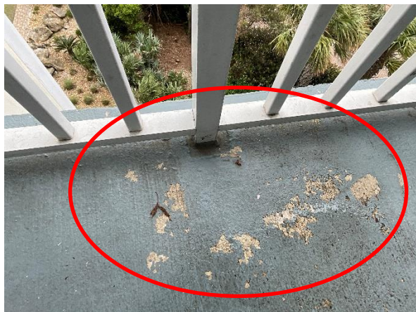
Photo 9 West Elevation – Private Balconies – Floor 4 – View of failed coating at concrete deck – Typical.
