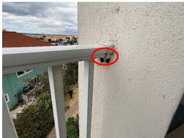
Photo 21 West Elevation – Private Balconies – Floor 3 – View of corroded side plate fasteners – Isolated.
