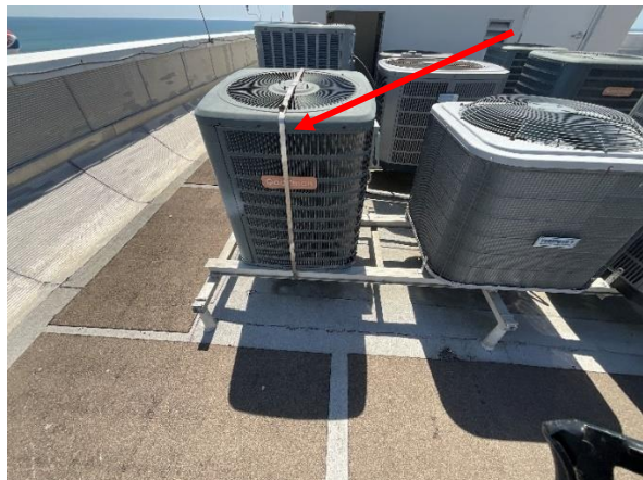
Photo 15 Roof – View of HVAC unit with poor support and no hurricane straps – Isolated.
