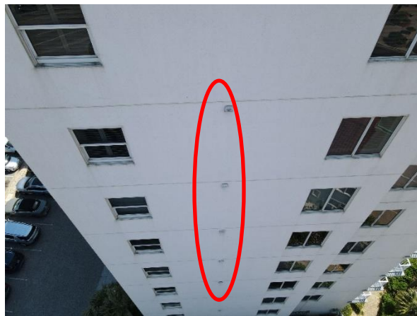
Photo 20 North Elevation – Overall View showing broken dryer vents – Typical.
