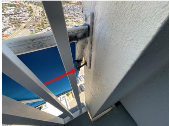
Photo 14 East Elevation – Common Walkways – Penthouse Floor – View of loose and corroded fasteners – Isolated.
