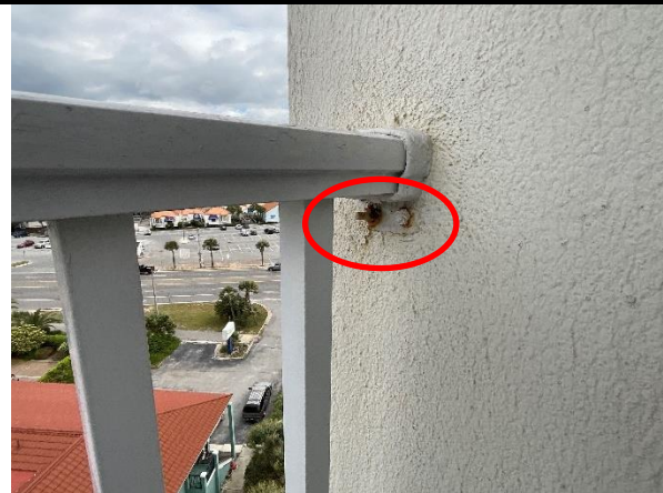
Photo 22 West Elevation – Private Balconies – Floor 3 – View of corroded side plate fasteners – Isolated.
