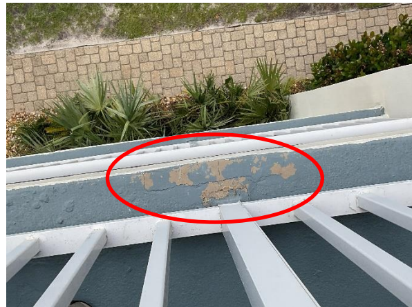
Photo 11 West Elevation – Private Balconies – Floor 3 – View of failed coating at concrete deck – Typical.
