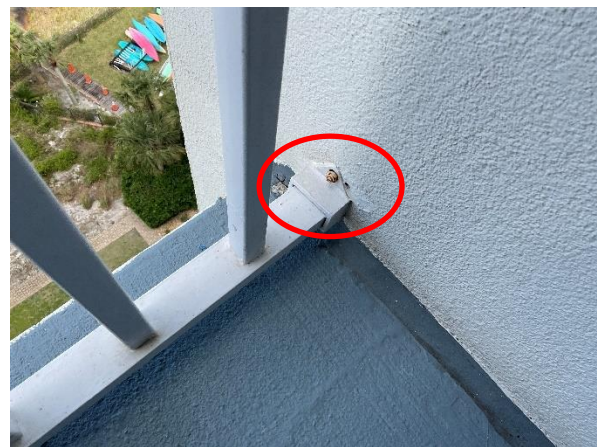
Photo 23 West Elevation – Private Balconies – Floor 10 – View of hole behind side plate fastener – Isolated.
