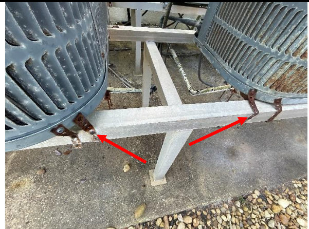
Photo 16 North Elevation – View of corroded hurricane straps – Typical.
