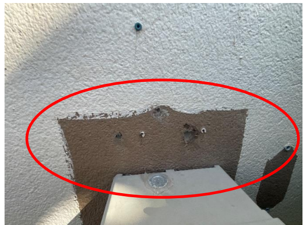
Photo 6 South Elevation – View of unpainted cladding unsealed abandoned fastener holes – Isolated.
