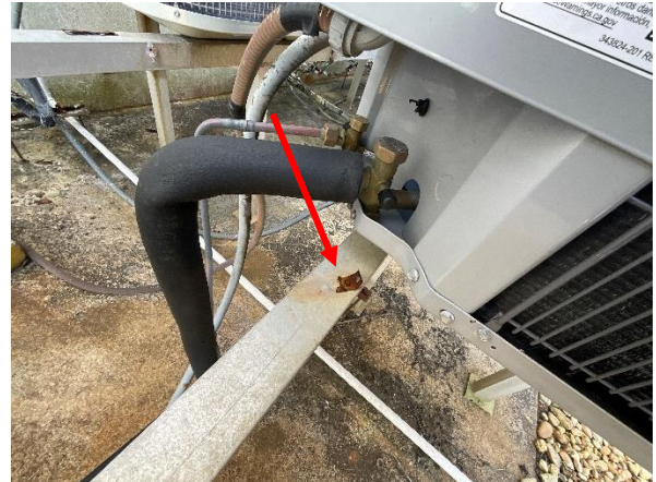
Photo 17 North Elevation – View of corroded and broken hurricane strap – Typical.
