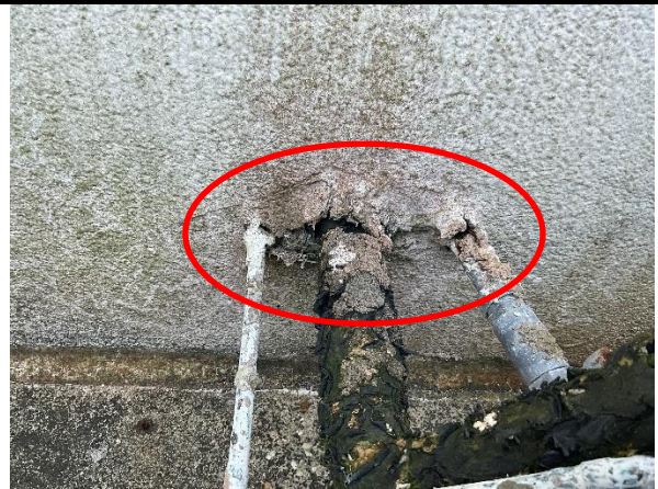
Photo 4 North Elevation – View of failed sealant at wall penetration – Isolated.
