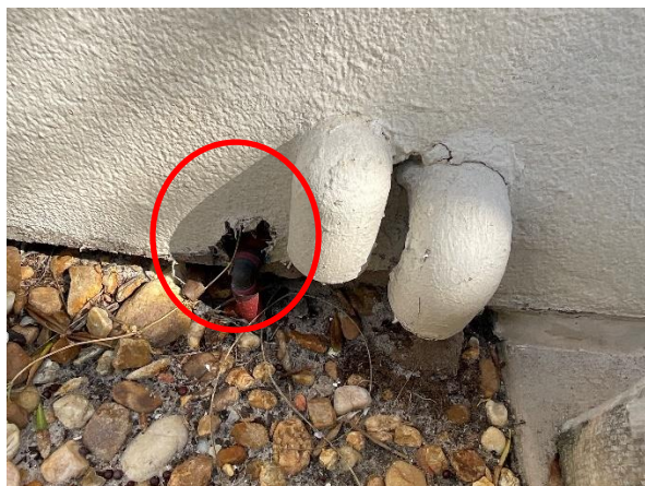
Photo 3 South Elevation – View of failed sealant at wall penetration – Isolated.
