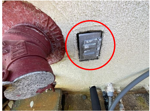
Photo 5 North Elevation – View of failed sealant at wall penetration – Isolated.
