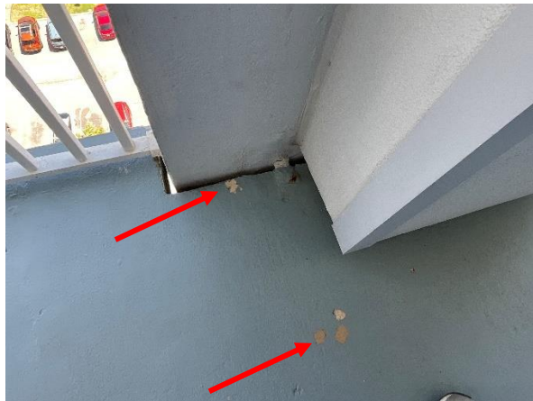
Photo 8 East Elevation – Common Walkways – Floor 11 - Overall View of failed coating at concrete deck – Typical.
