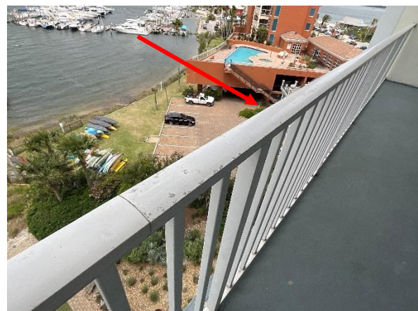
Photo 24 West Elevation – Private Balconies – Floor 6 – View of loose top rail – Typical.
