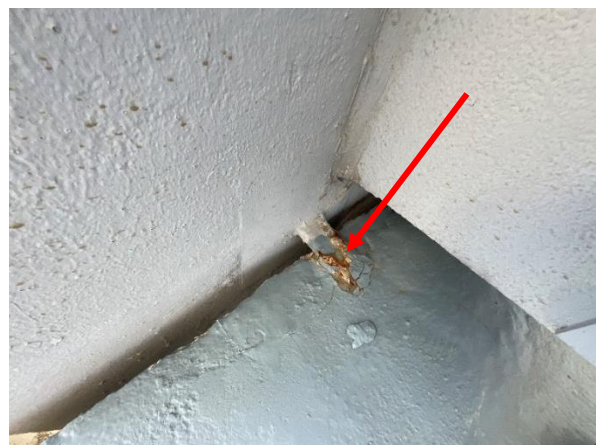
Photo 12 East Elevation – Common Walkways – Floor 5 – View of corroded knee wall tab – Typical.
