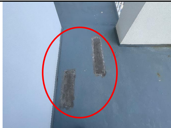
Photo 10 West Elevation – Private Balconies – Floor 13 – View of uncoated spall repairs on balcony deck – Typical.
